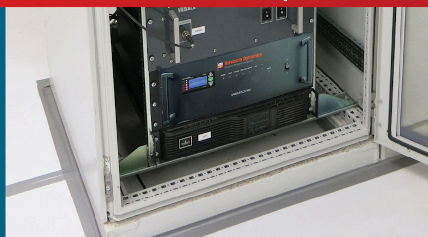
A fixed installation on the server rack on Banyu Urip FPSO
